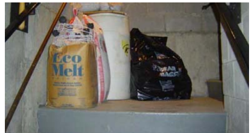
This photo is an example of materials being stored on a stair landing. Storing items on stair landings restricts the walkway, increasing the chances of slips and falls to occur.
