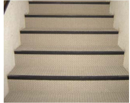
This photo is an example of carpeted steps that have been installed with a rubber nosing. The rubber nosing will protect the carpeting, keeping it from fraying or tearing and help make the stair nose visible.
